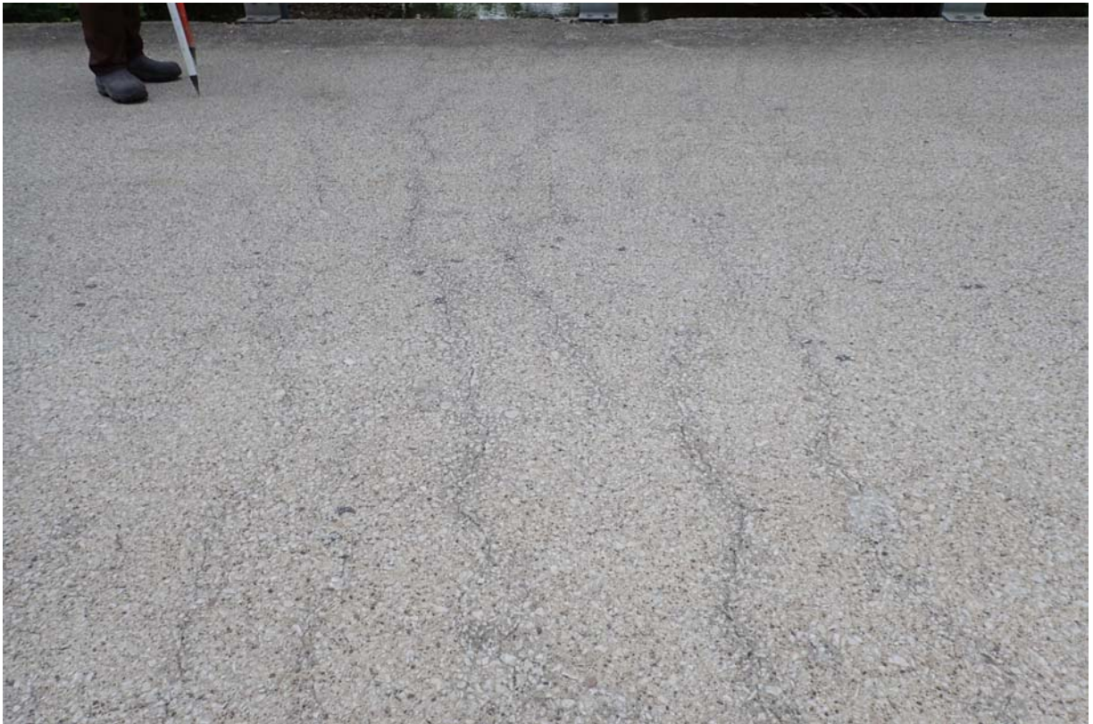
View of several minor sized transverse cracks in the wearing surface over the pier.
