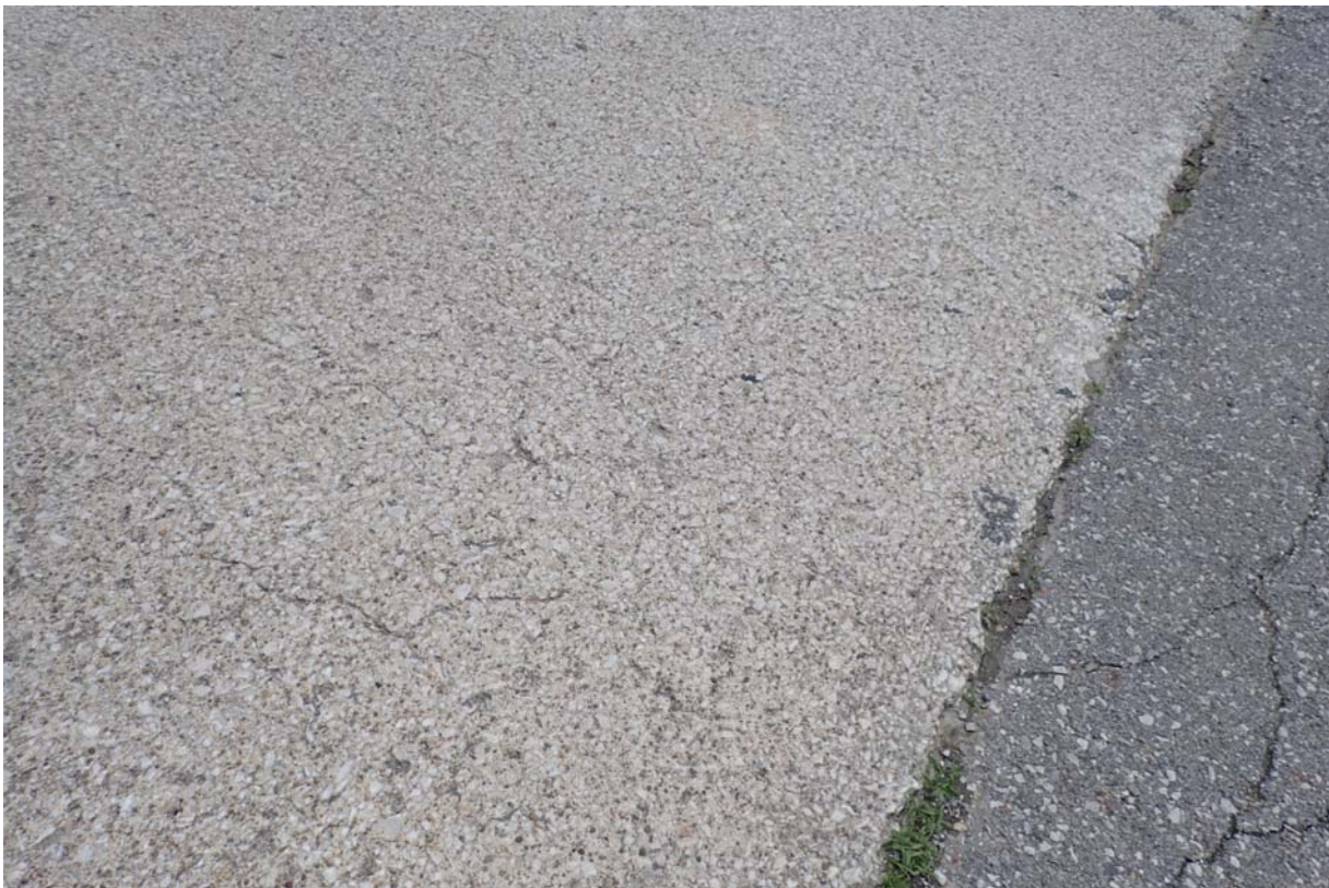
View of several minor sized cracks at the downstream south end of the wearing surface.
