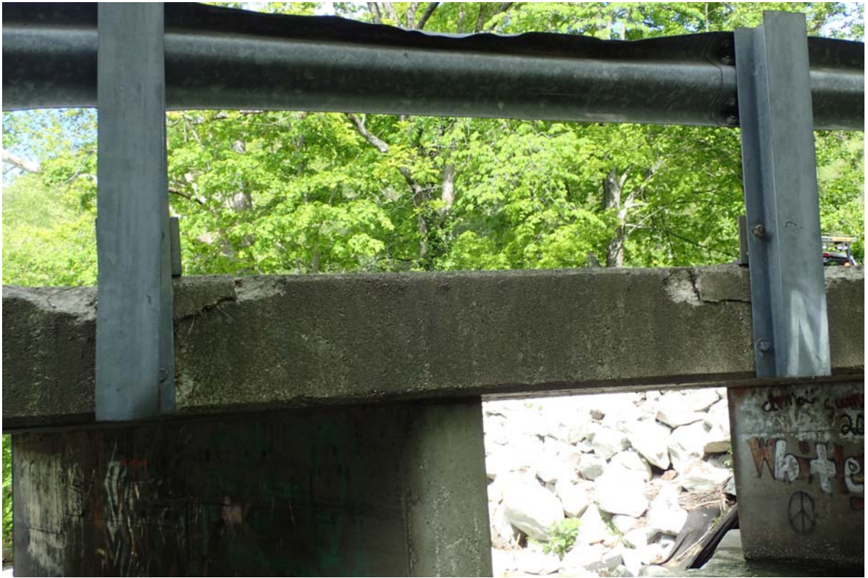
View of moderate spalls in the upstream face of the deck at rail post 4 and 5 from the south.
