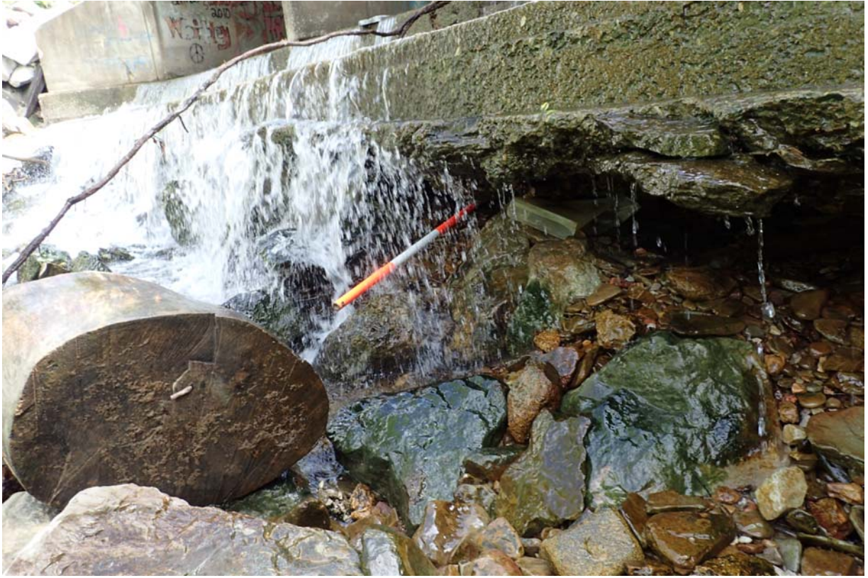
View of ~ 7.5'-8' of horizontal undermining at the south end of the protection apron.
