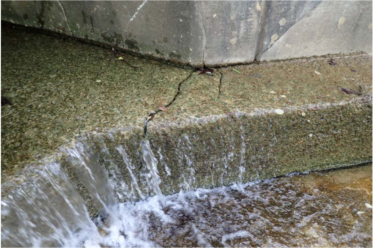
View of full depth cracking in the footing of the downstream south wingwall.
