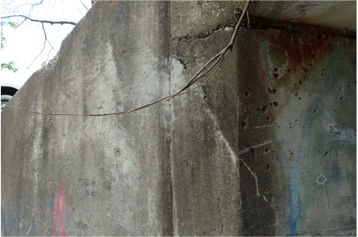
View of some minor cracking at the outlet end of the north abutment.
