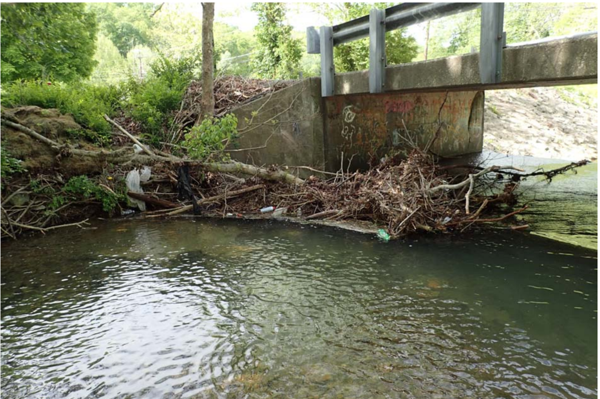
View of a moderate drift pile at the inlet end of the south span.
