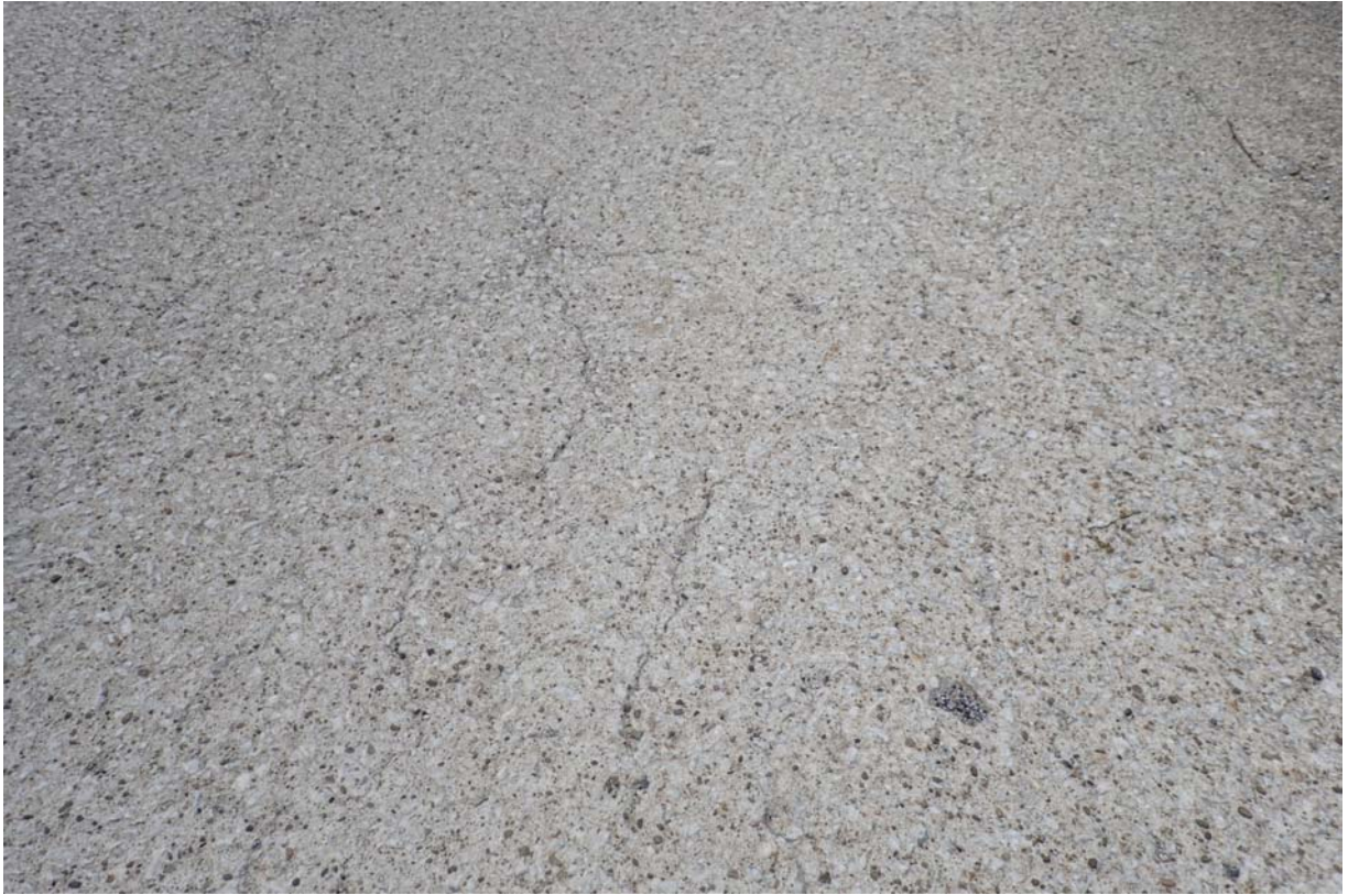
View of several longitudinal cracks at the downstream north end of the wearing surface.
