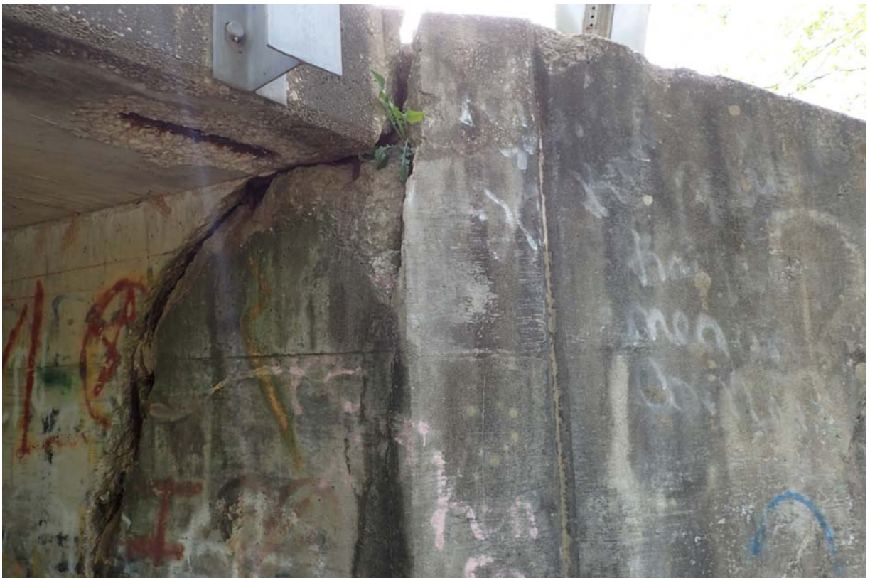
View of large heavy cracking and spalling with exposed steel at the downstream end of the south abutment. This cracking measures ~ 4.5" -5" wide at mid-height. Notice the cracking extends up through the top of the wingwall.
