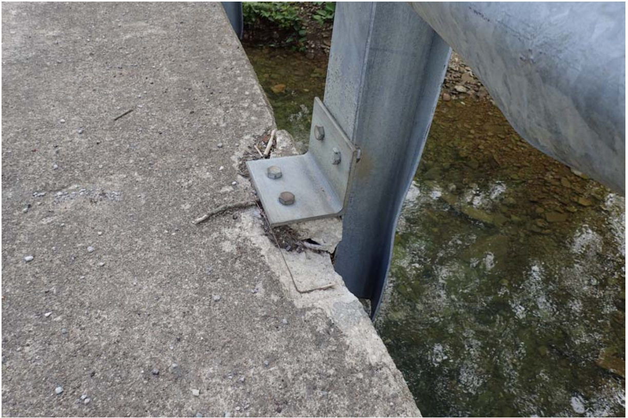
View of moderate cracking and spalling at upstream rail post 4 from the south.
