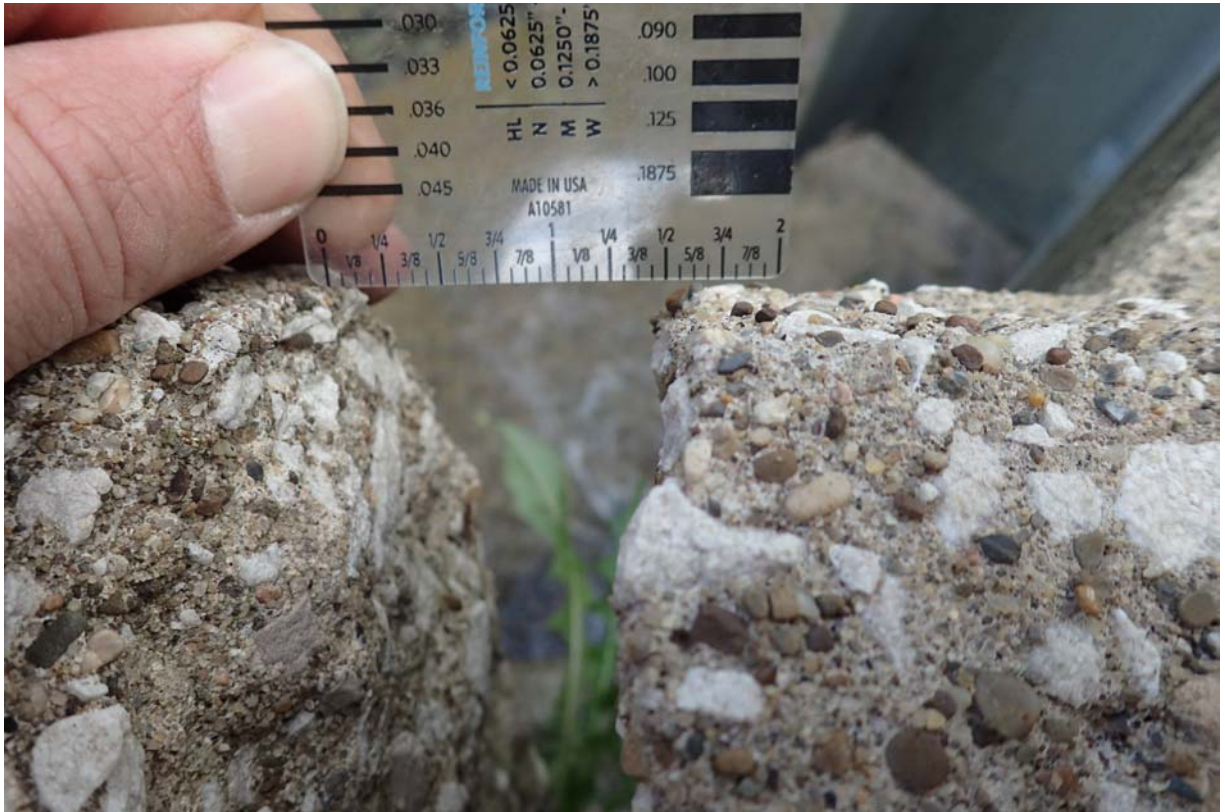
View of ~ 1.5" of separation at the top of the downstream south wingwall.
