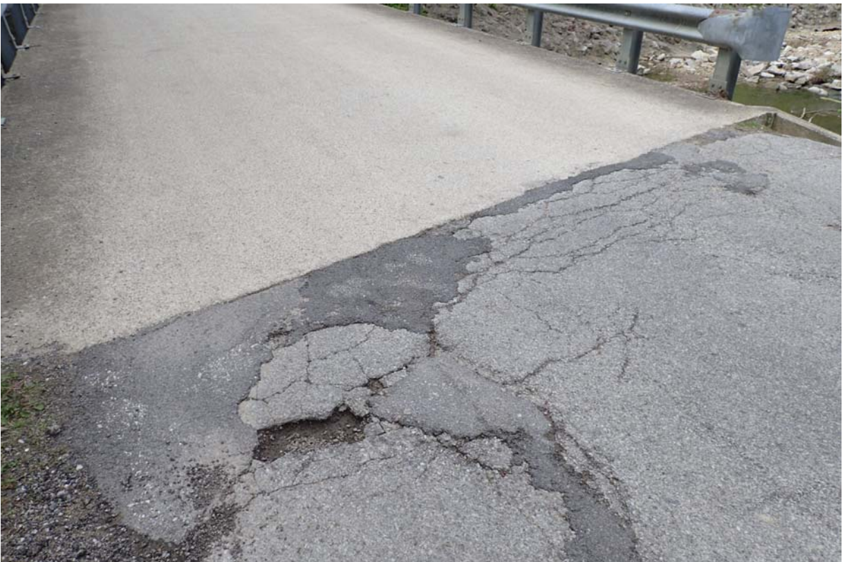
View of moderate cracking, potholes, and patching along the north approach.
