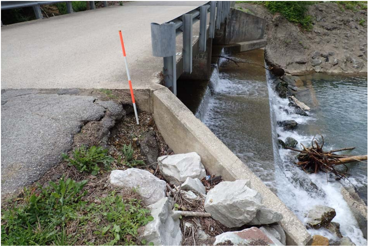
View of moderate erosion at the downstream north wingwall. Notice the roadway shoulder is breaking up.
