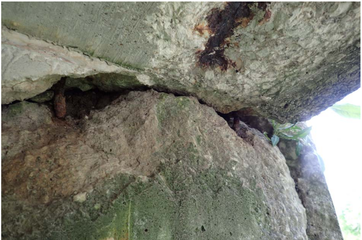
View of large heavy cracking and spalling with exposed steel at the top downstream end of the south abutment/slab interface.
