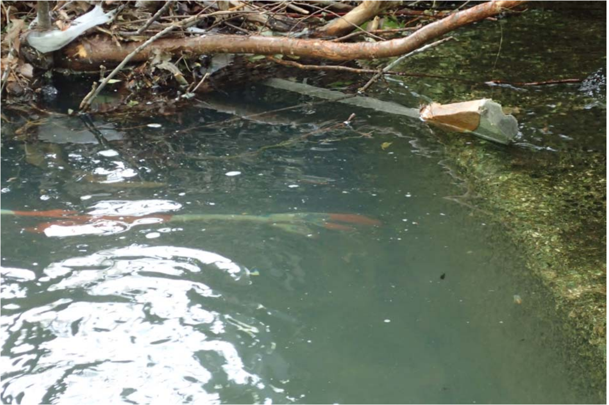
View of ~ 18" of horizontal undermining under the inlet floor of the south span.
