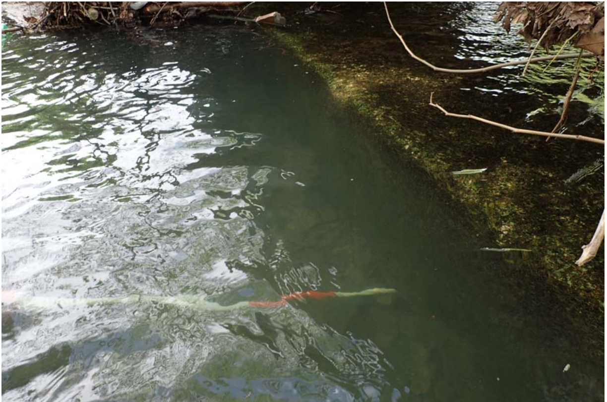
View of ~ 12" of horizontal undermining under the inlet floor of the south span.
