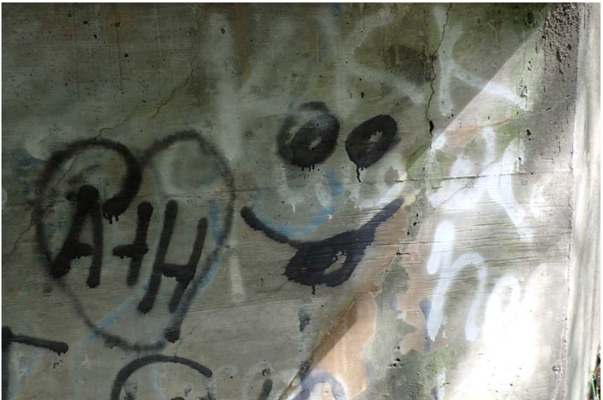
View of some minor cracking at the inlet end of the north abutment.
