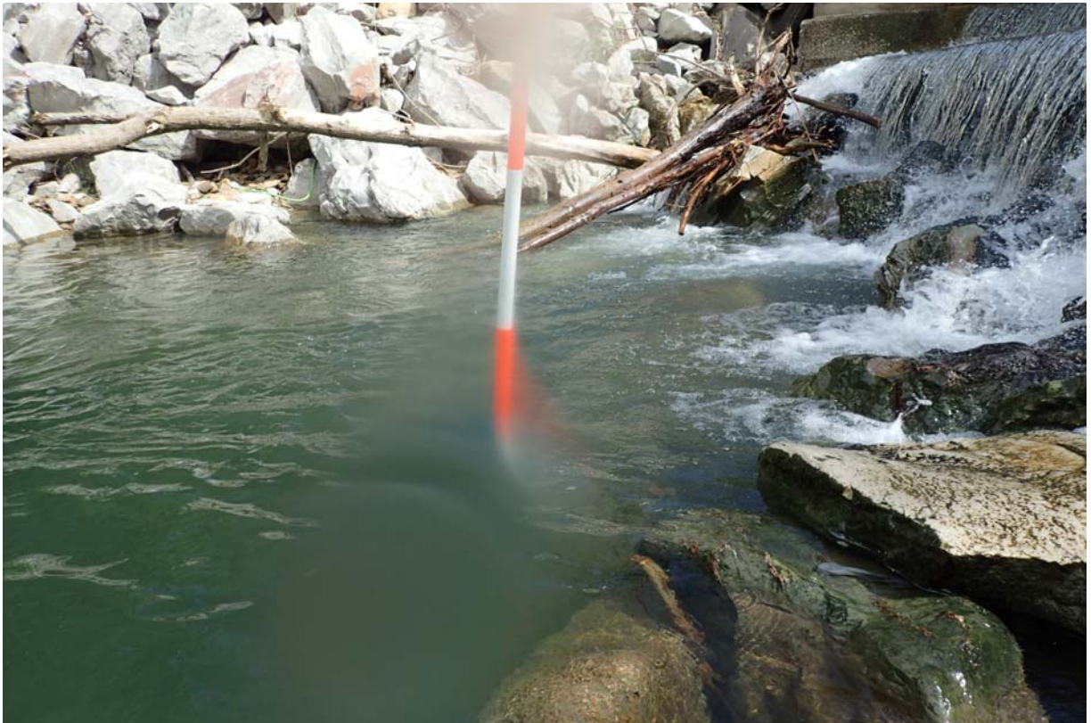
View of ~ 3' deep scour hole below the protection apron.
