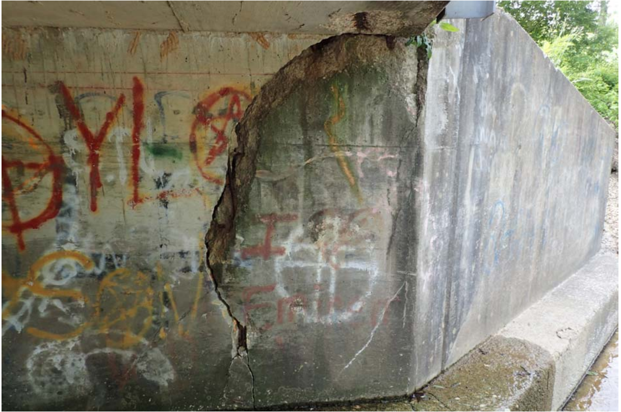
View of large heavy cracking and spalling with exposed steel at the downstream end of the south abutment. This cracking measures ~ 4.5"-5" wide at mid-height.
