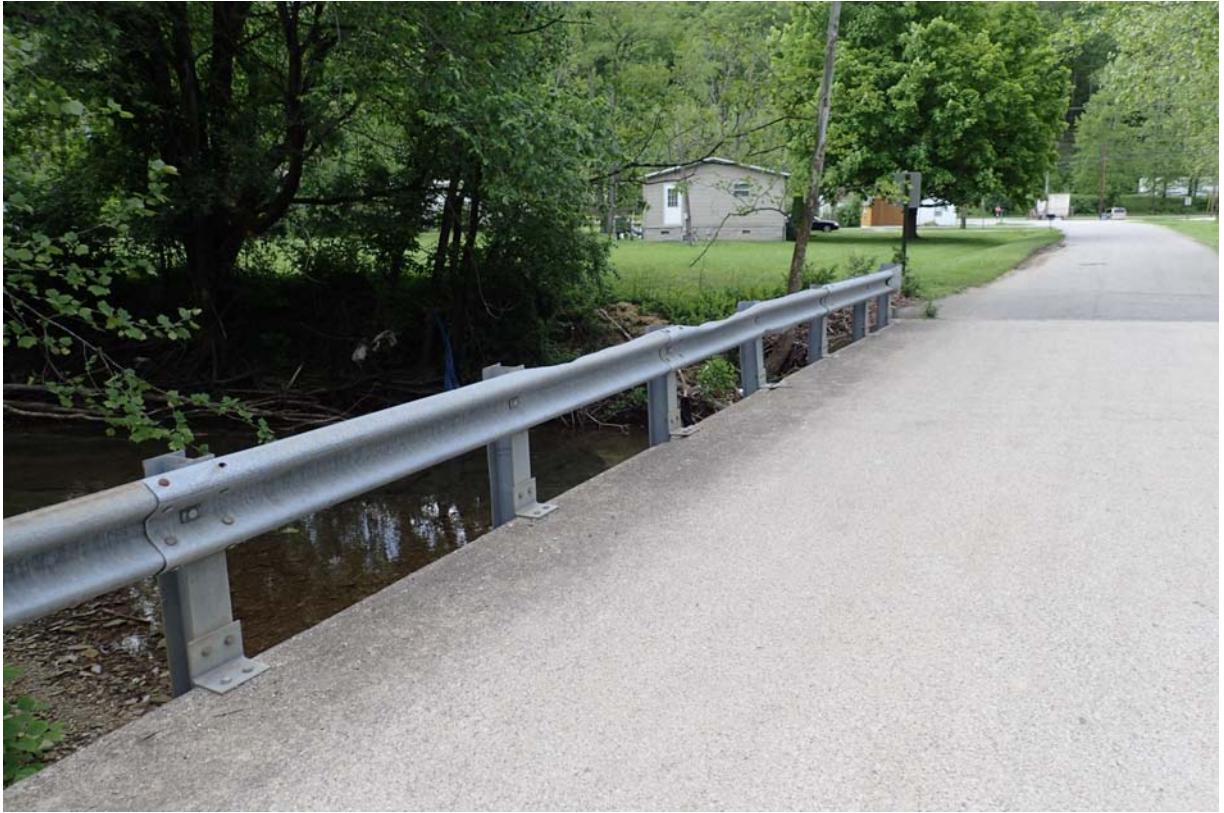
View along the upstream railing. Notice the moderate impact damage near mid-length.
