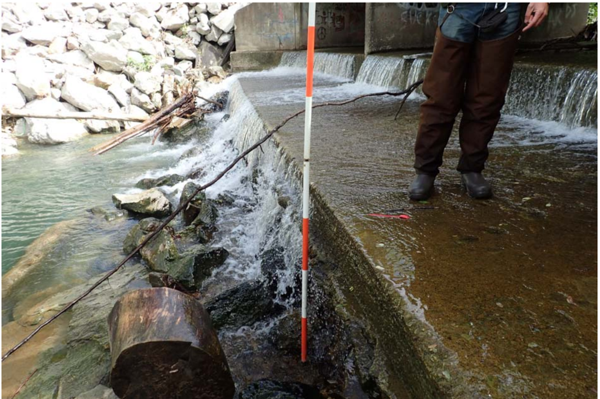
View of the ~ vertical drop off the protection apron.
