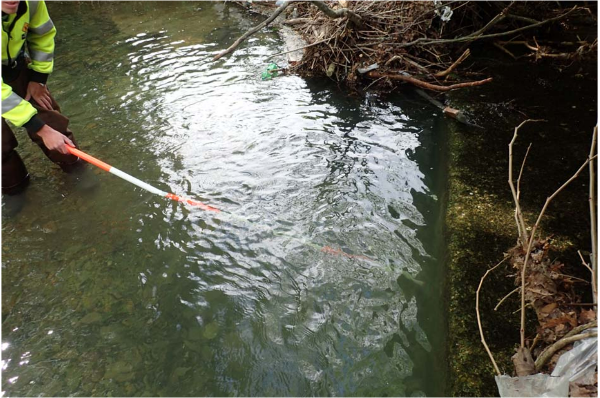
View of ~ 12" of horizontal undermining under the inlet floor of the south span.
