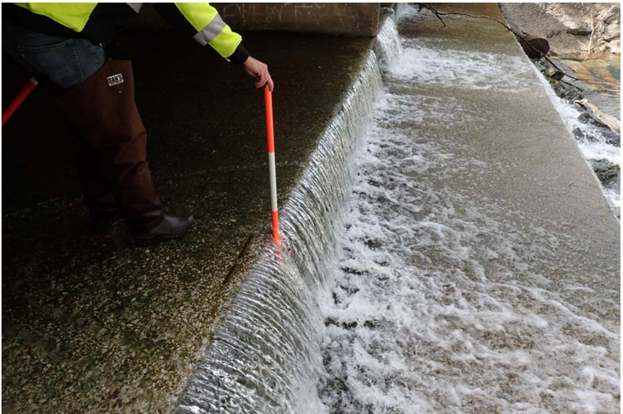
View of an ~ 18" vertical drop of the floor in the north span.
