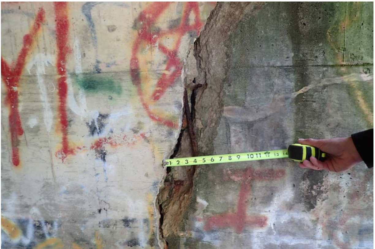
View of large heavy cracking and spalling with exposed steel at the downstream end of the south abutment. This cracking measures ~ 4.5"-5" wide at mid-height.
