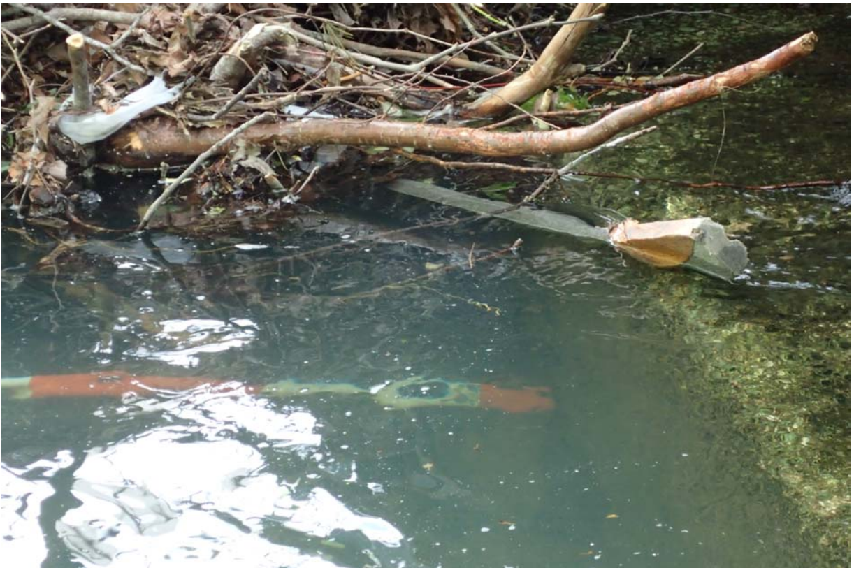
View of ~ 12" of horizontal undermining under the inlet floor in the south span.
