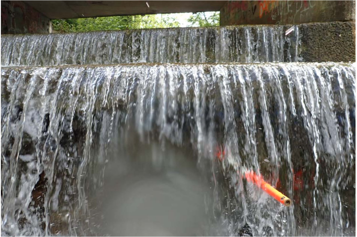
View of ~ 6.5' of horizontal undermining at the north end of the protection apron.
