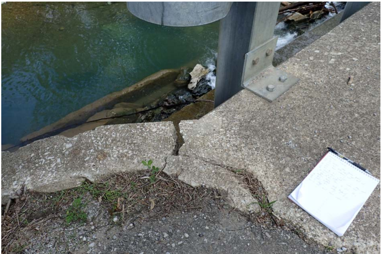
View of ~ 1.5" of separation at the top of the downstream south wingwall.
