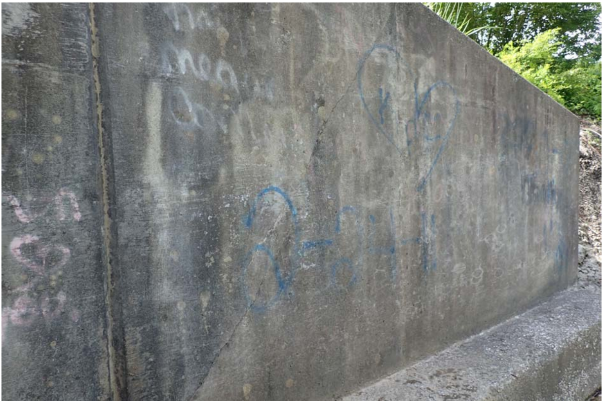
View of a minor sized full height diagonal crack in the downstream south wingwall.
