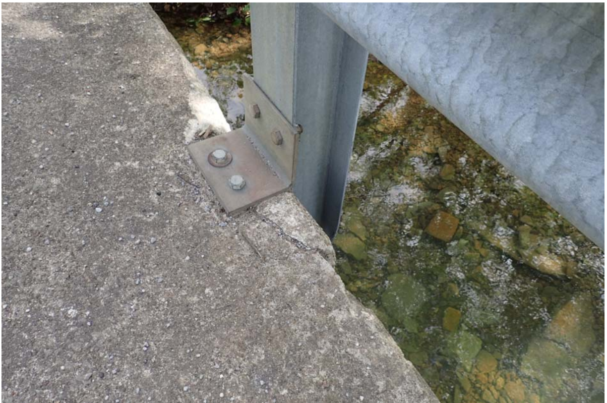
View of moderate cracking and spalling at upstream rail post 5 from the south.
