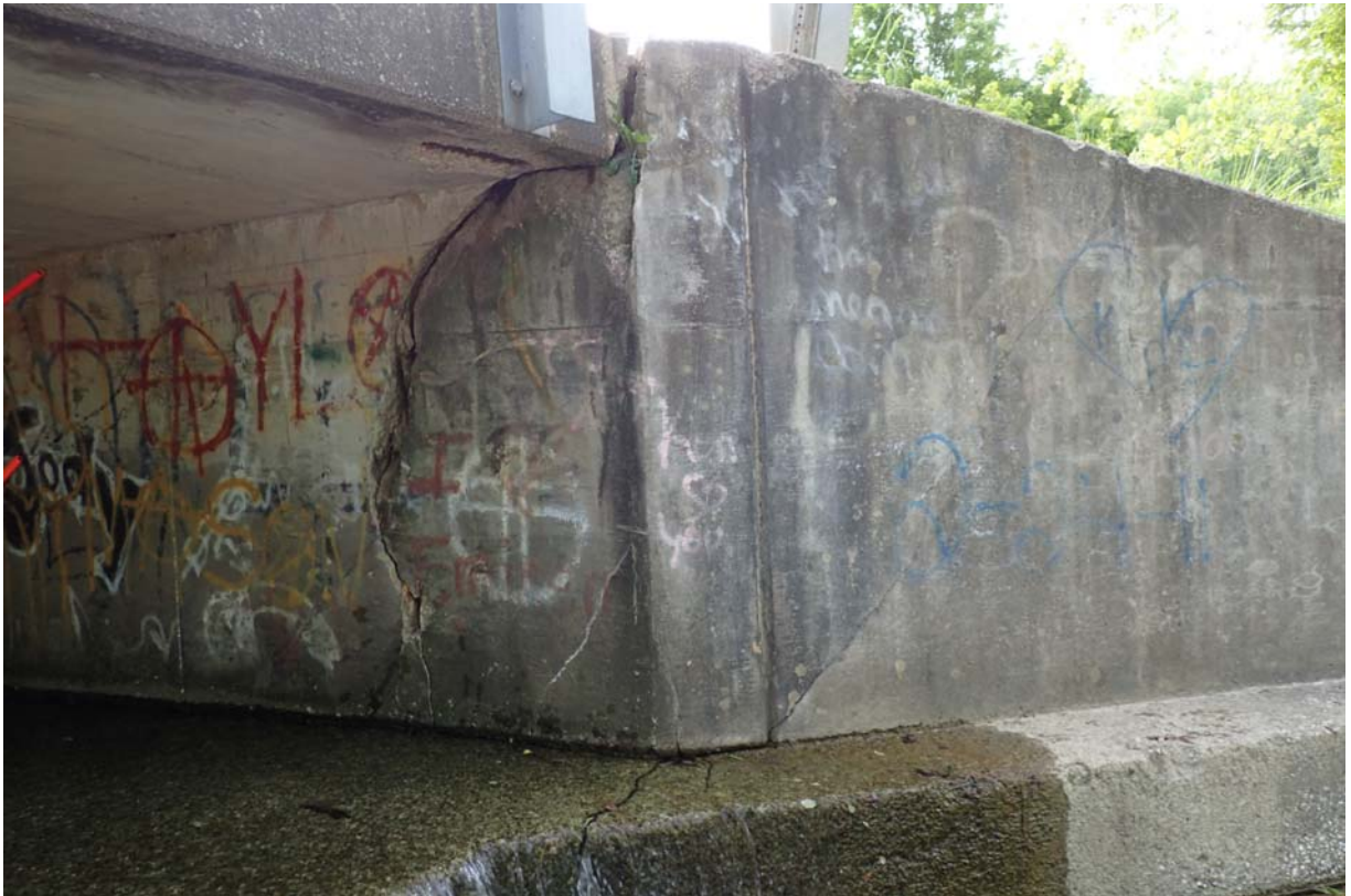
View of large heavy cracking and spalling with exposed steel at the downstream end of the south abutment. This cracking measures ~ 4.5" -5" wide at mid-height. Notice the cracking extends from the bottom of the footing to the top of the wingwall.
