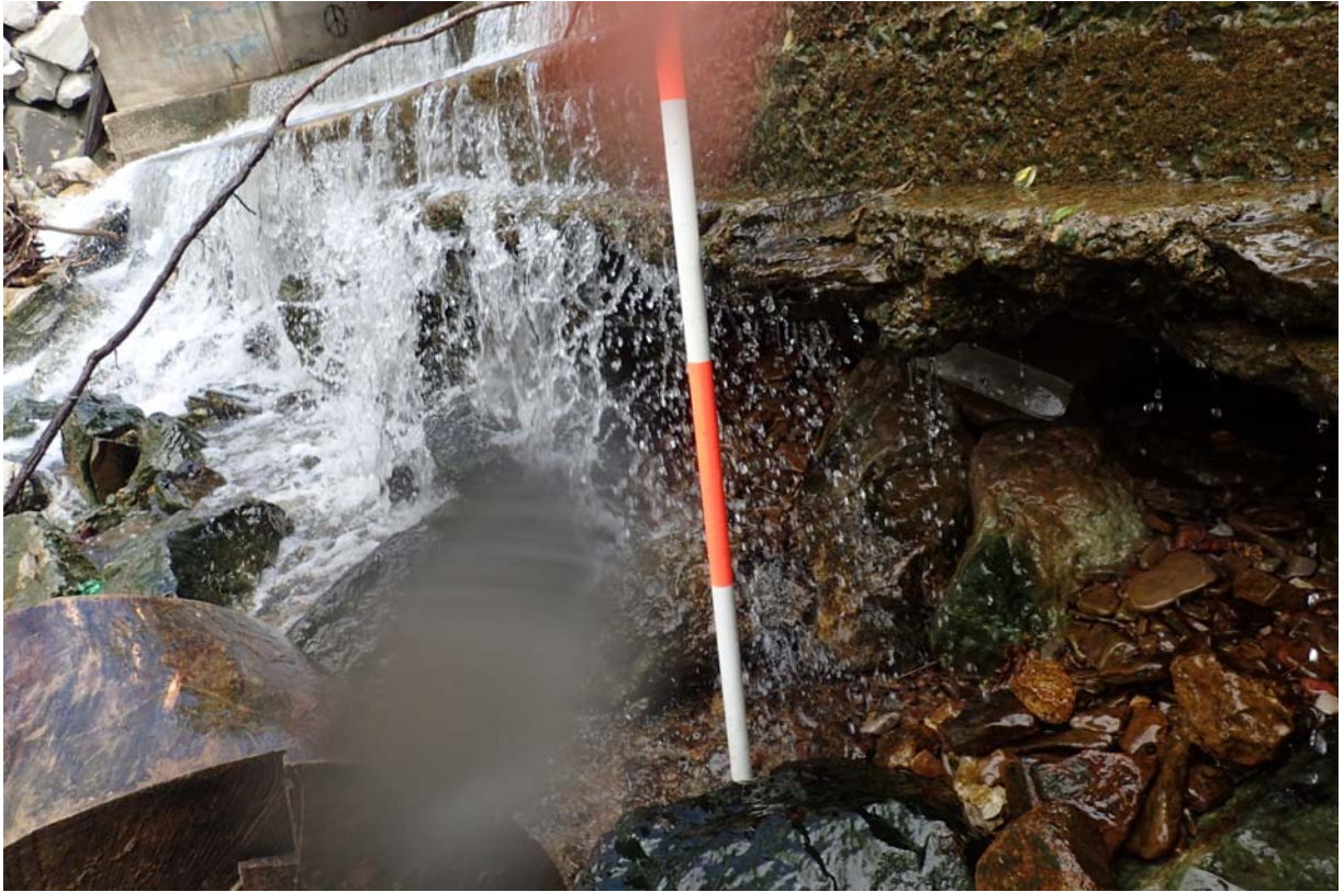
View of ~ 2'-2.5' of vertical undermining of the protection apron.
